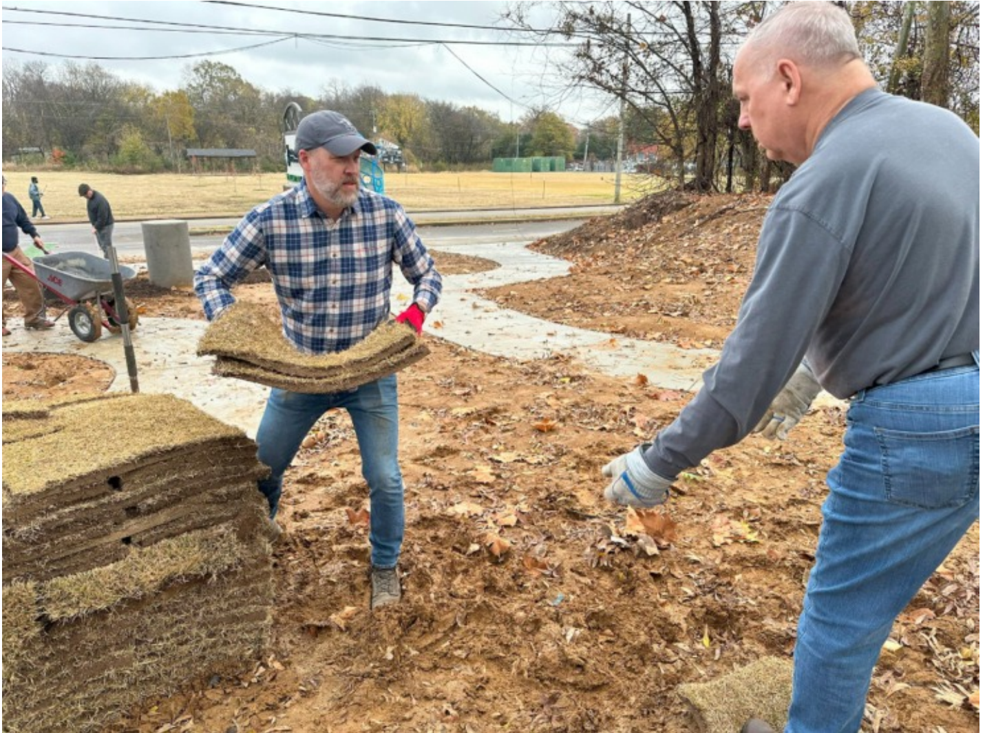
Carpenter Art Garden and a team of collaborators are constructing Tillman Sculpture Park on the corner of Princeton Avenue and Tillman Street. (Courtesy Brandon Herrington)
